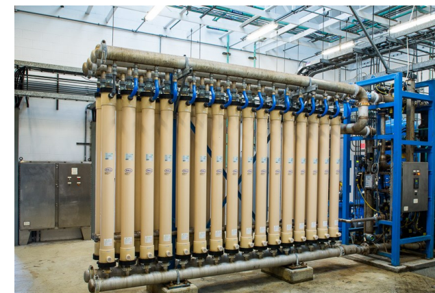
Youngs River Lewis & Clark Treatment Plant
